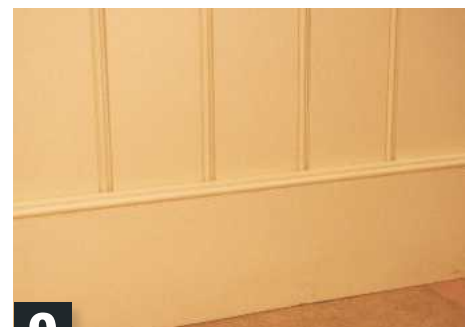
9 Finished skirting and panelling is neat with concealed fixing, though easy to remove for access
